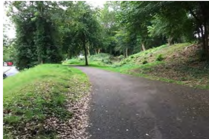
Steep gradient and perched path above Clifton Down road makes The Promenade unsuitable as a consistently shared route for pedestrians and cyclists
