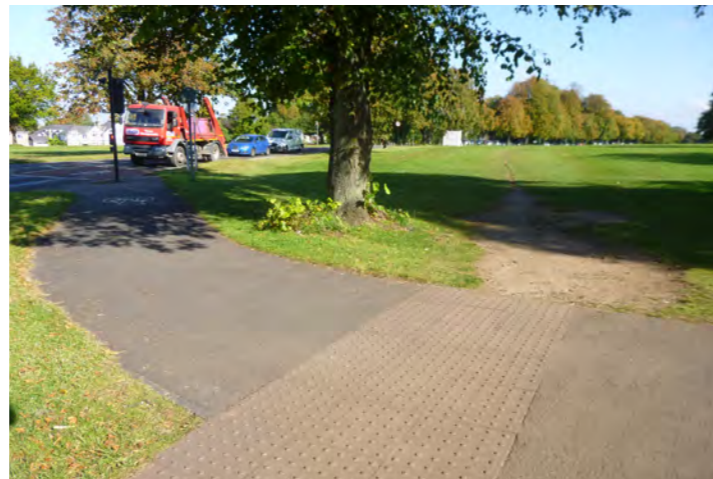
Poor connection of cycling and walking routes at key junctions leads to erosion of adjoining grass
