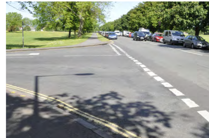
Large radius corners on side roads encourage high vehicle speeds and makes crossing difficult for pedestrians. There are inconsistent or no dropped kerbs
