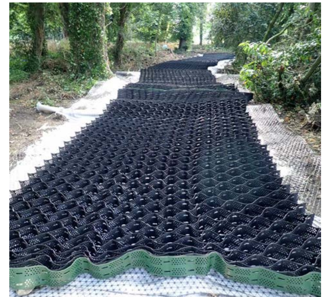
Construction and finished path through Wormside Wood (Grade II Listed), part of the Waddesdon Greenway Project 2018
